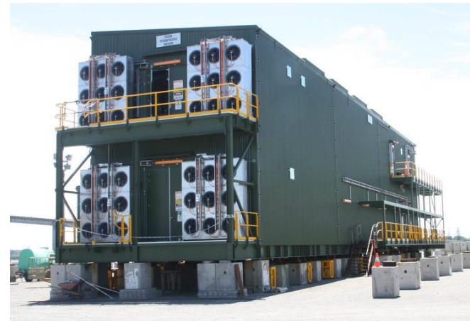
Mine site E-house
