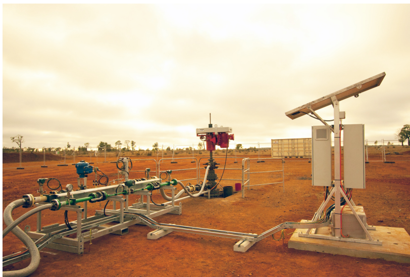
Oil field pump station
