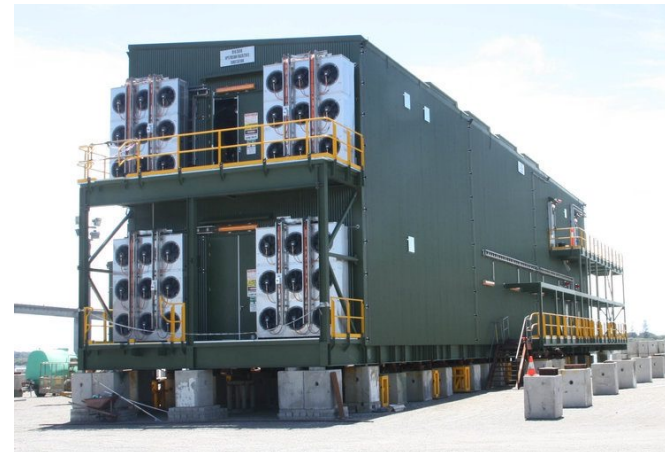
Mine site E-house
